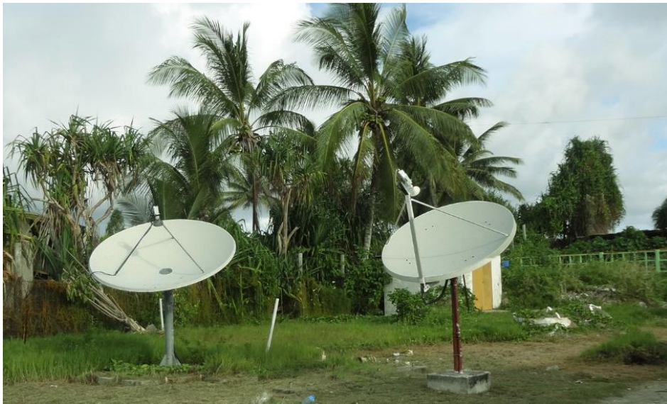
Receive Station for J-SAT C-band satellite Himawari (left) Speedcast Ku-band VSAT antenna for Speedcast network (right)
